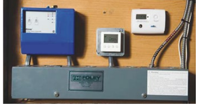
Additional controls inside the Mendota's boiler room.
